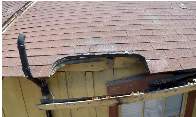
Figure 1-10 Hagemann Farm Roof and Gutter Condition
