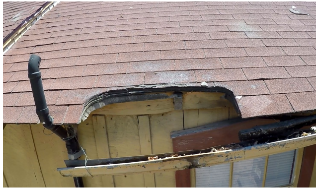
Figure 1-10 Hagemann Farm Roof and Gutter Condition
